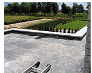
An EPDM rubber roof
