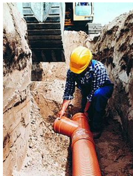
PVC is used extensively in sewage pipes due to its low cost, chemical resistance and ease of jointing
